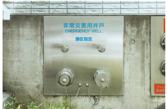
Emergency water well (rendition)
