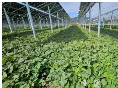
Mori Building Tochigi City Miyamachi Agricultural Solar Power Plant
