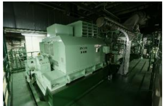
Gas engine generator (rendition)
