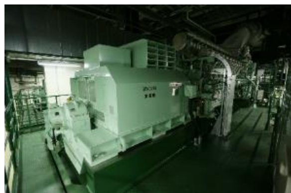
Gas engine power generator
